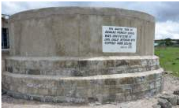
Primary School Water Tank, Kenya. Source: Aidlink
